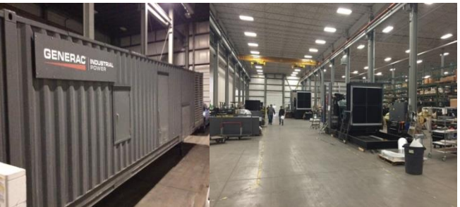
LARGE INDUSTRIAL GENSET LINE OSHKOSH, WI
